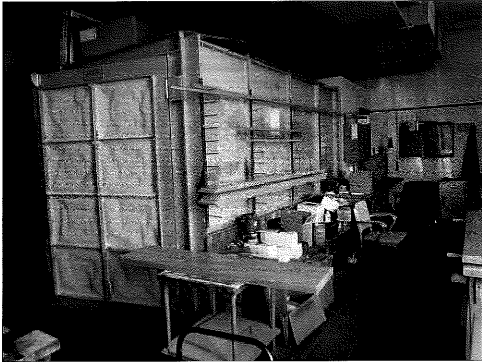
Spray booth in paint room
