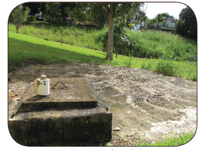
Keep septic tanks sealed.
