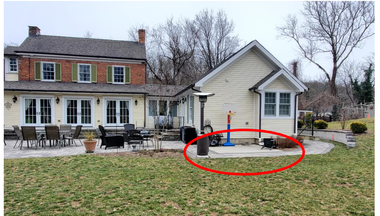
Figure 36: Existing concrete pad to be bordered in Nicolock pavers. Existing walkway in front of concrete pad to be removed (Item 26).
