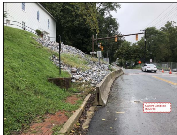
Figure 12: St. Luke AME Church slope after the 2016 flood.
