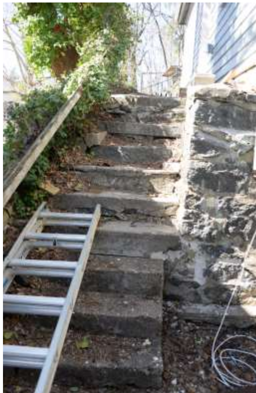
Figure 43 – Concrete and granite stairs to be all granite
