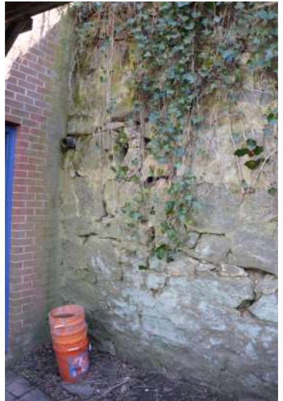
Figure 57 - Historic wall to be repaired
