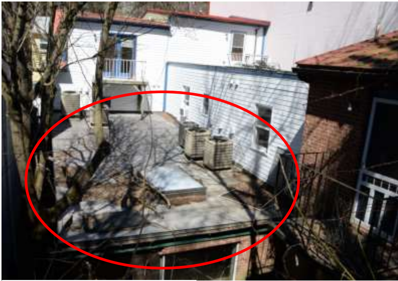
Figure 56 - Roof to be replaced
