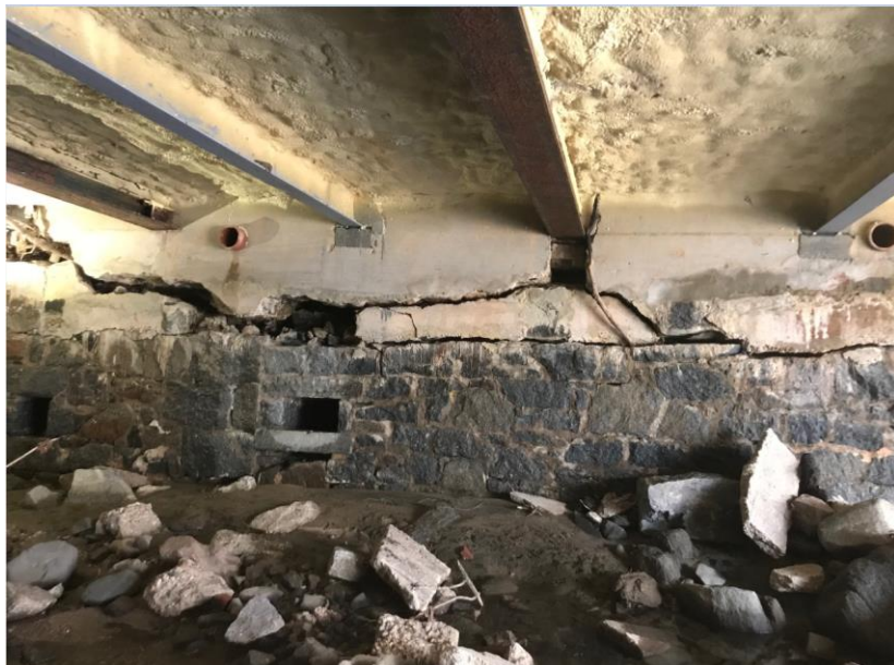
Figure 6 - View of foundation/rear wall separation underneath building in stream channel
