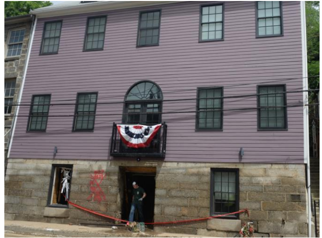
Figure 2 - Building after the 2018 flood
