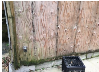
Figure 31 - Plywood at 8181 Main Street
