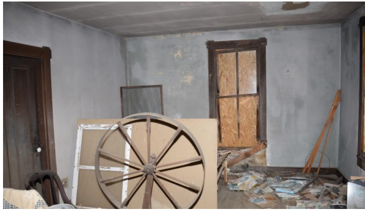
Figure 19 - Interior view showing damage to window
