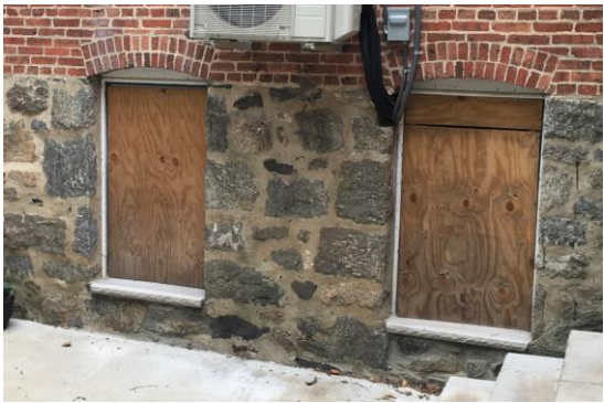
Figure 27 - Boarded up windows at 8173 Main Street
