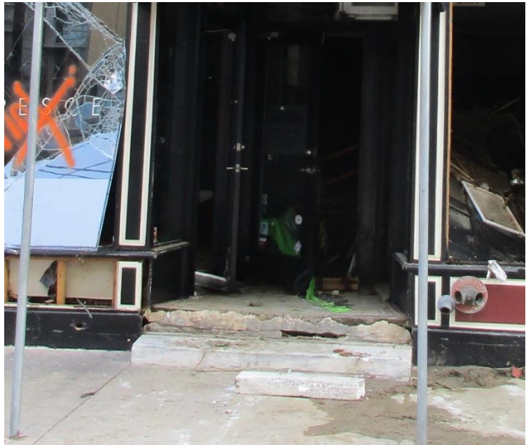
Figure 6 - Condition of entry after flood
