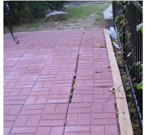
Figure 25 - Previously constructed patio without approval that was destroyed in flood
