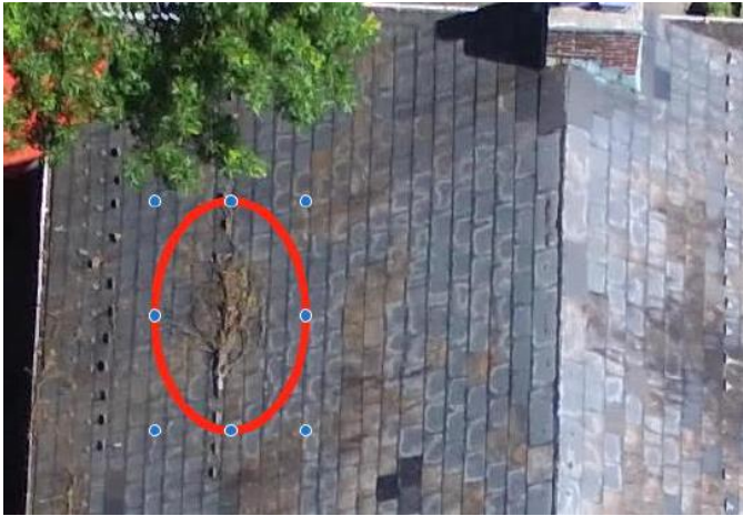
Figure 11 - Aerial view of roof damage.
