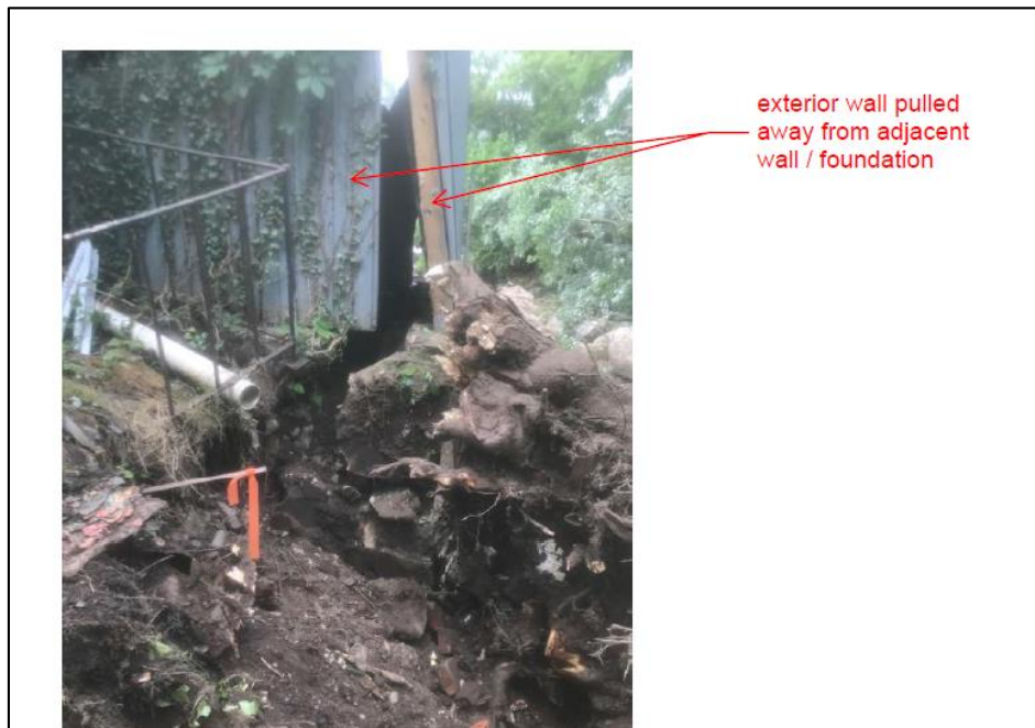
Figure 2 - View looking west at tree root and damage to lean-to
