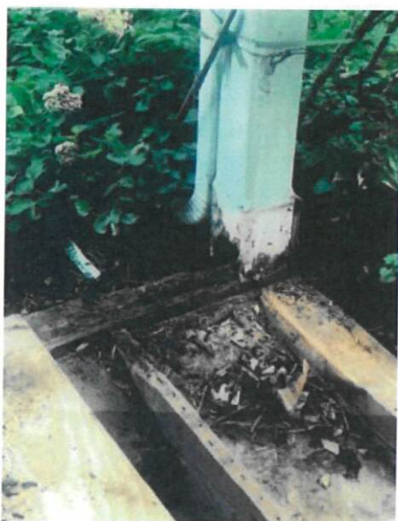
Figure 10 - Example of rot on porch.
