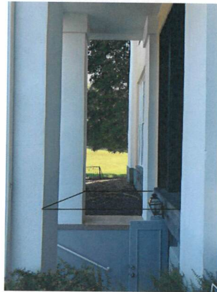
Figure 7 - Northwest elevation where first floor porch will be reconstructed. Note black square outlining area of porch. Granite stairs to flank each side of the porch.
