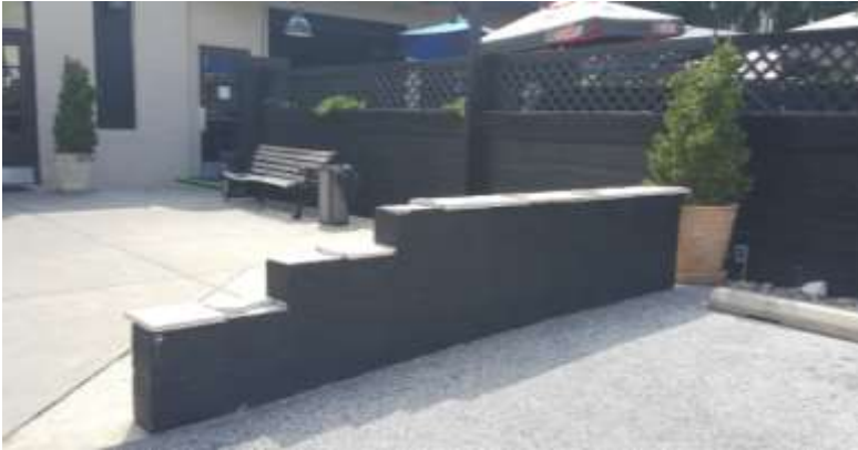
Figure 9 - Before - Original block wall that was proposed to be replaced with a wall
