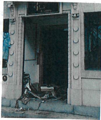
Figure 35 - Damage from 2016 flood
