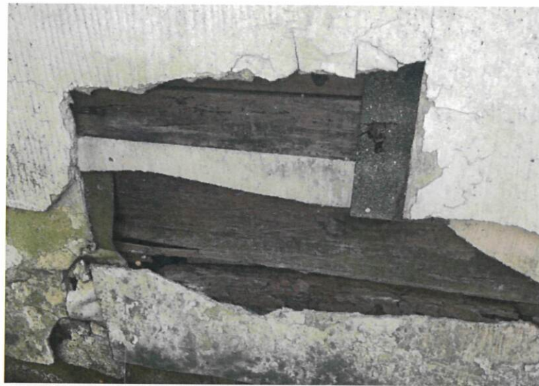
Figure 5 - Wood visible under asbestos.
