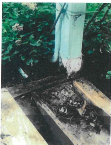
Figure 10 - Example of rot on porch.
