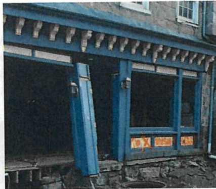
Figure 33 - Damage from 2016 flood
