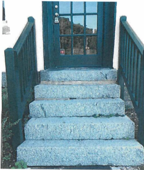
Figure 6 - Existing service entry steps and railing. To be matched on new steps and railing.
