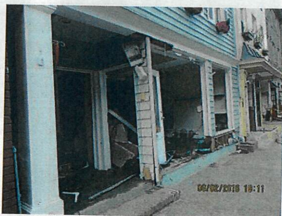
Figure 27 - Damage from 2016 flood
