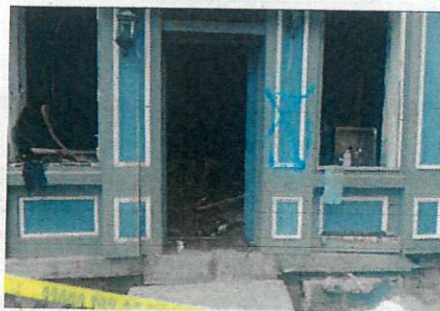
Figure 40 - Damage post 2018 flood
