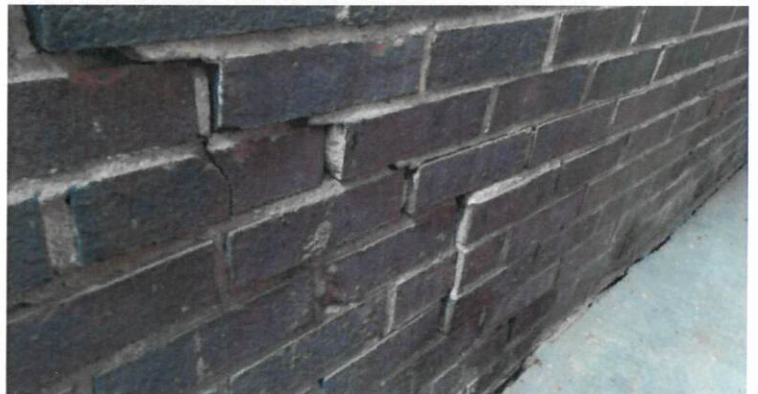
Figure 14 - Damage to existing wall.
