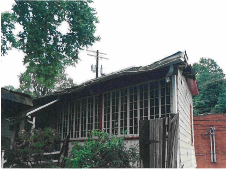
Figure 8 - Damage to rear of building
