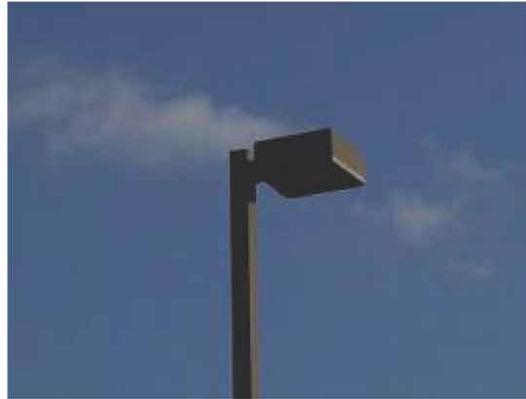
INTERNAL SITE LIGHTING
