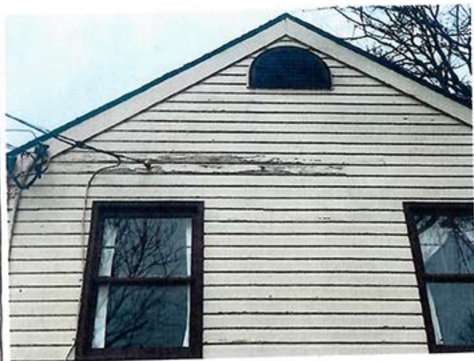
East End of P388 Court Ave Paint Peeling
