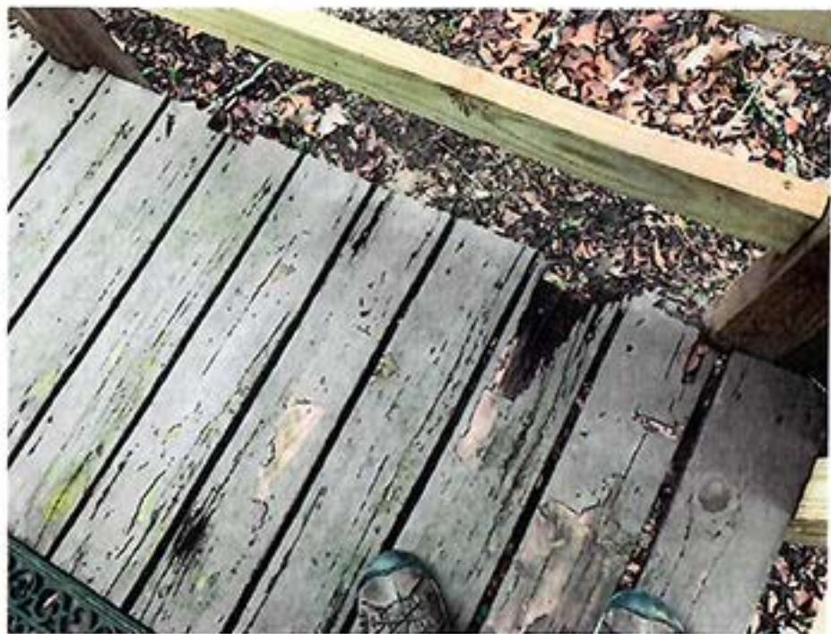
8388 Court Ave Rear Entrance, Deck boards rotten
