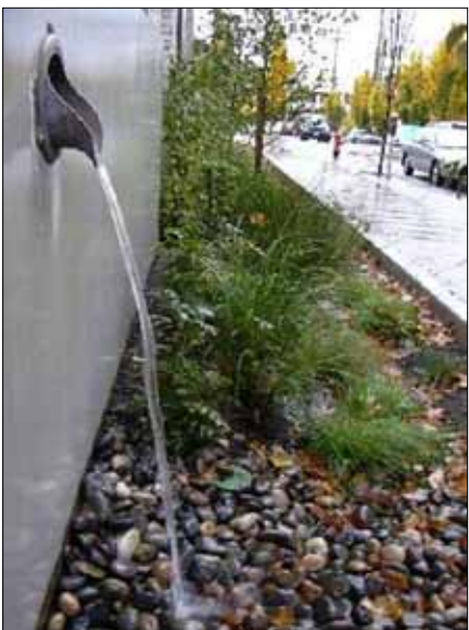
Rooftop Stormwater Treatment
