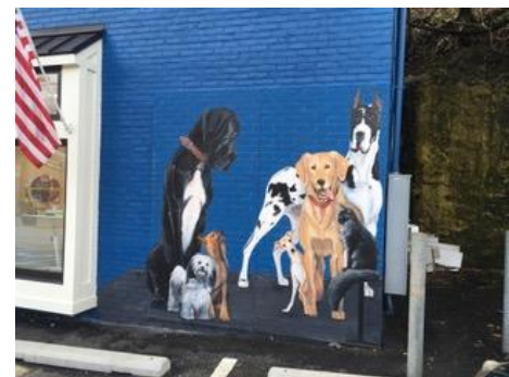
Figure 22 - Mural installed without approval
