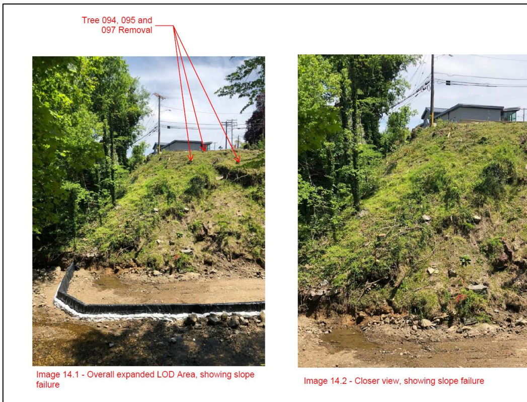
Figure 18 - Area of slope failure and T-94, T-95 and T-97 removal, picture from application
