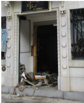
Figure 35 - Damage from 2016 flood
