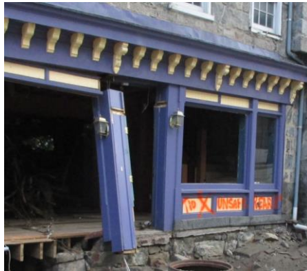
Figure 33 - Damage from 2016 flood
