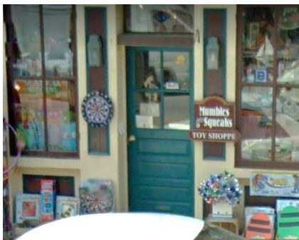
Figure 39 - Previously existing door prior to 2016 flood
