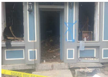
Figure 40 - Damage post 2018 flood
