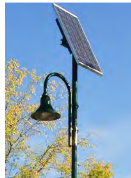
Solar Powered Lighting Source: Philips Hadco Lighting
