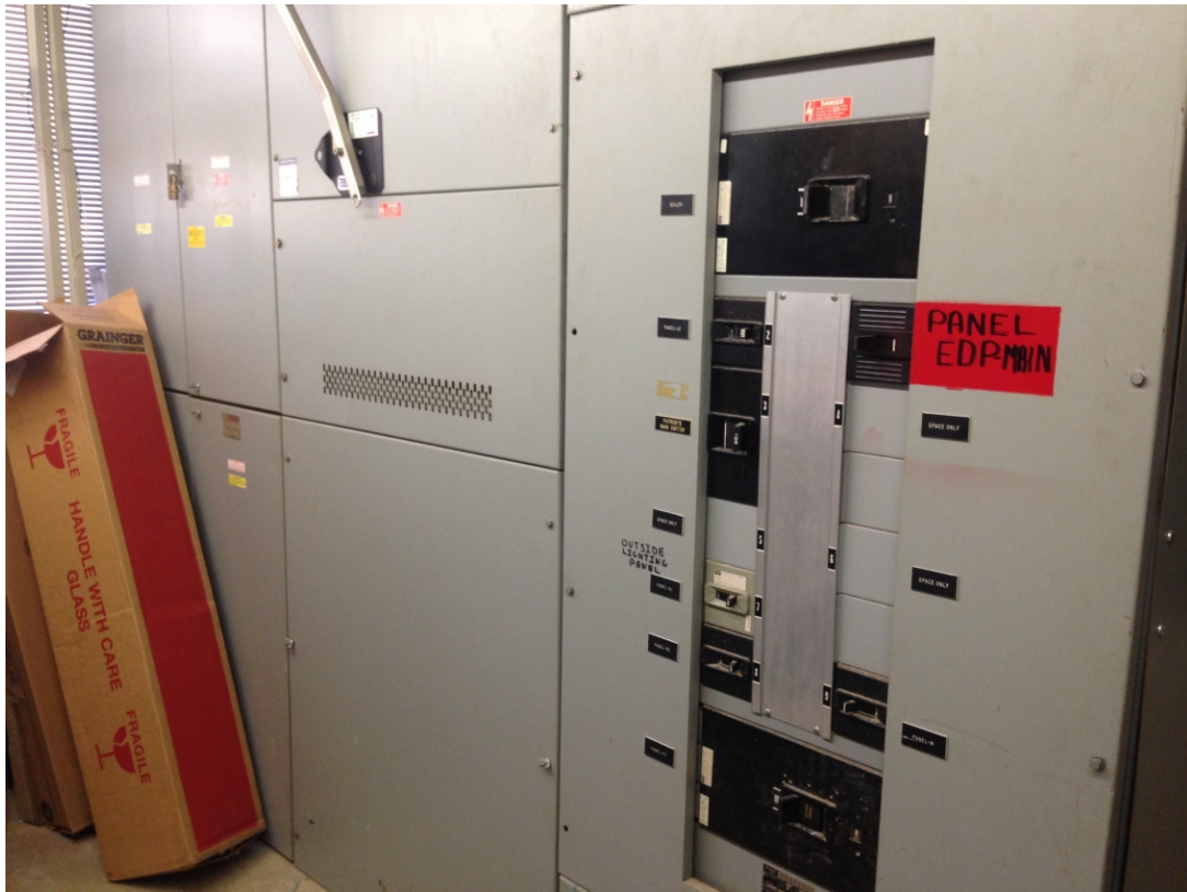
Photo 7: View of the electrical room located on the first floor of the on-site building.
