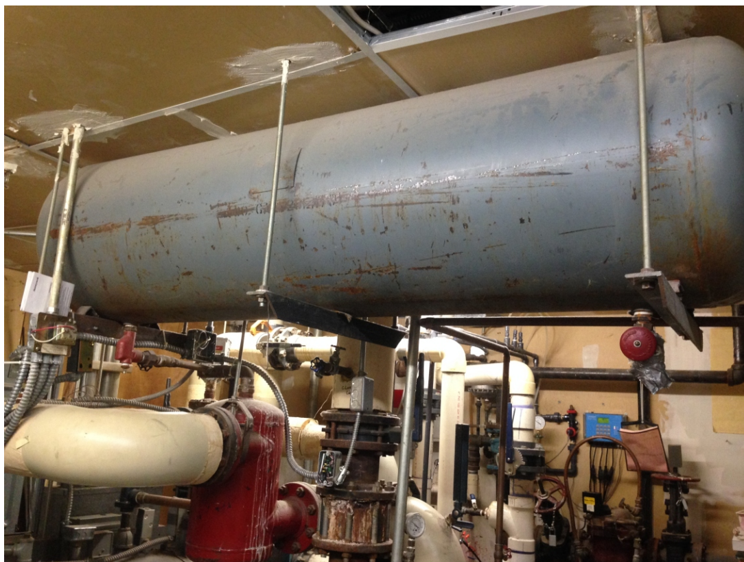
Photo 8: View of the boiler room located on the first floor of the on-site building.
