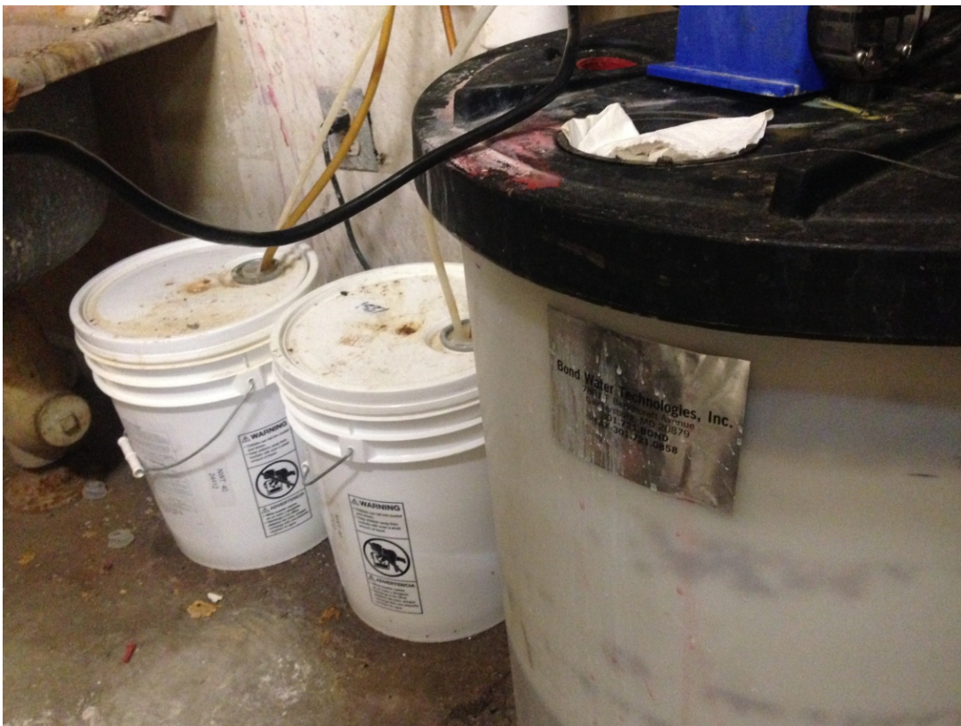
Photo 10: View of the containers of Bond 125 located in the boiler room.
