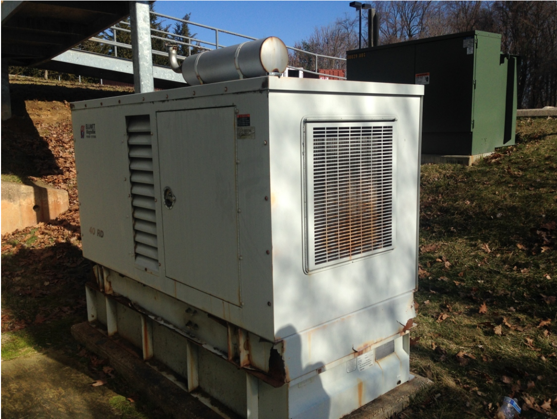
Photo 5: View of the diesel-fueled generator located outside the northern portion of the on-site building.
