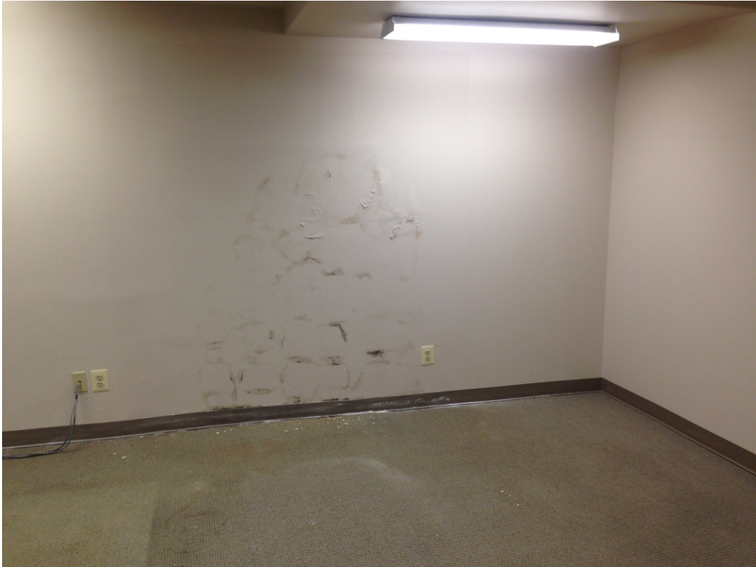
Photo 11: View of one of several rooms where visible mold growth was observed during the site inspection.
