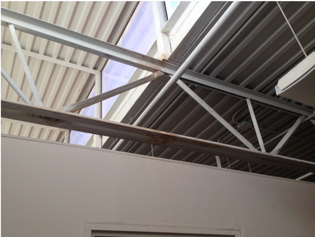
Photo 12: View of one of several locations where indications of water intrusion were observed during the site inspection.
