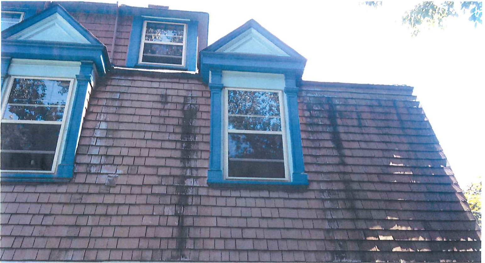
DAMAGED SHINGLES WALL RIGHT SIDE
