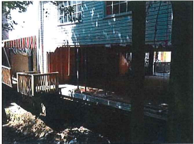
Rear of 8129 after removal of 7/2016 flood debris and destroyed first floor wall. Prior deck after removal of compressor and existing rear windows.
