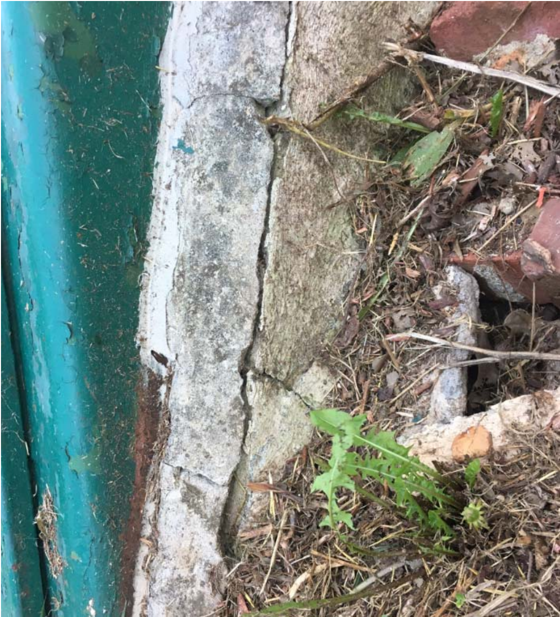
External view of cellar door- cracks in foundation
