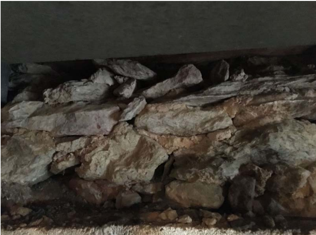
Foundation wall, masonry degraded
