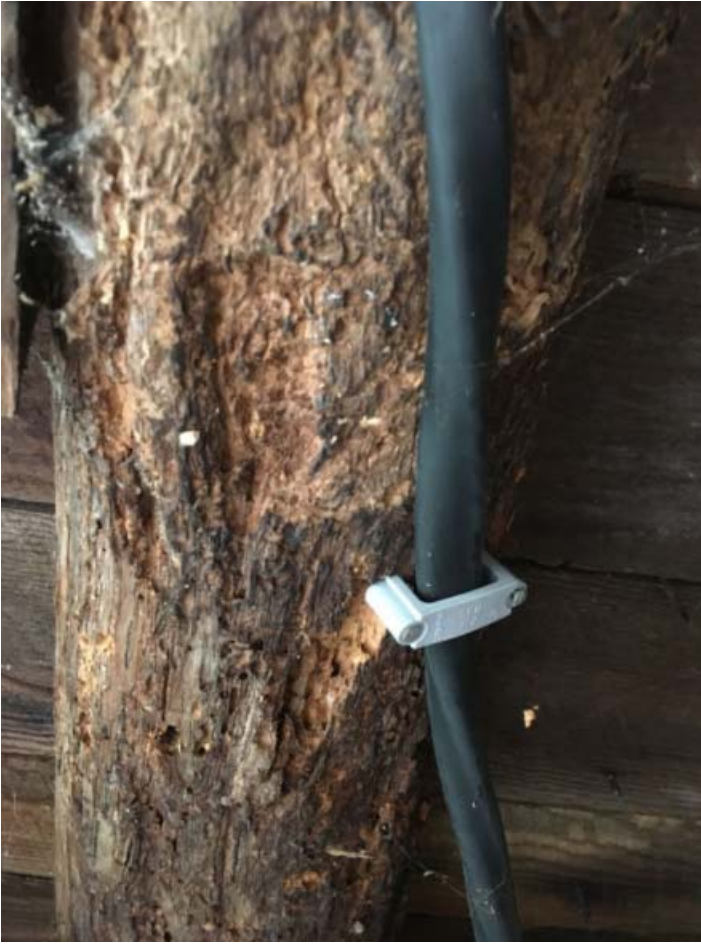
Bug damaged joist
