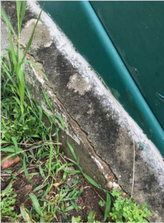
Large crack, exterior of Bilco doors
