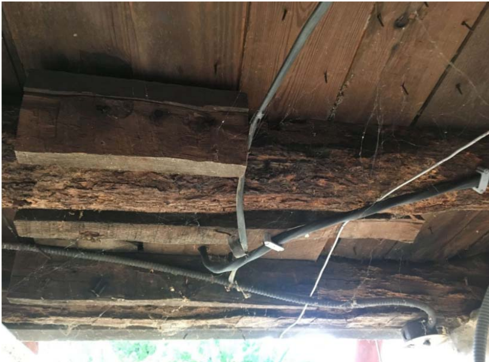
Bug damaged joist near exit
