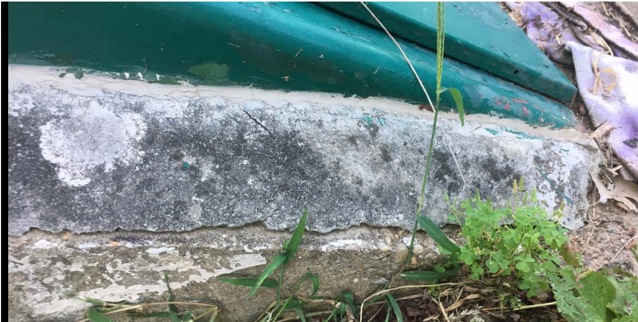
Outside of cellar door. Note large crack along frame. No longer connects to cement foundation.
