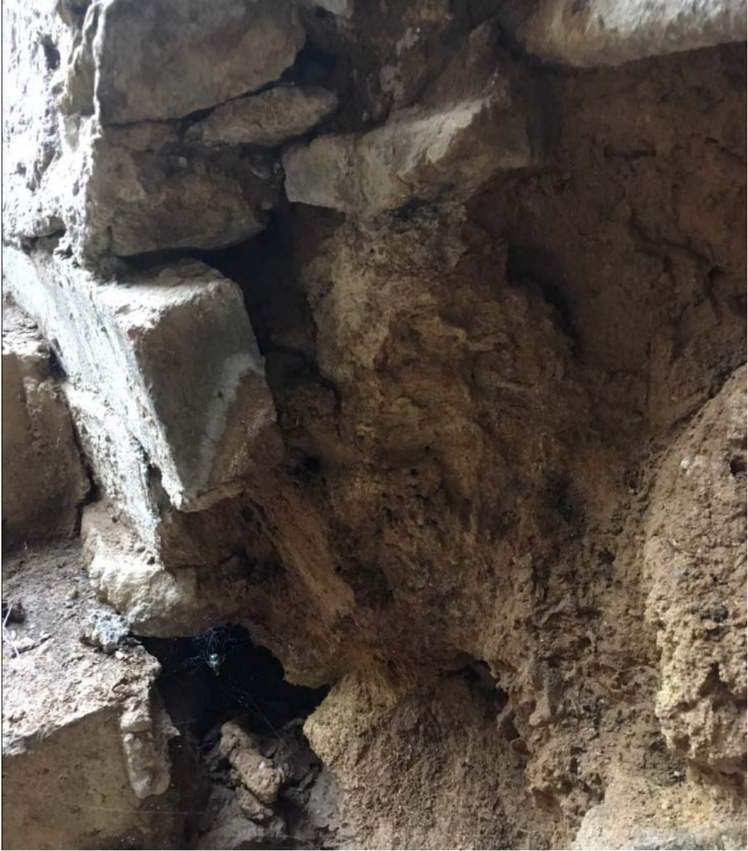
Closer view of crumbling foundation wall by entry way. Note bulging, loose bricks and stones. Also note holes where water comes in.
