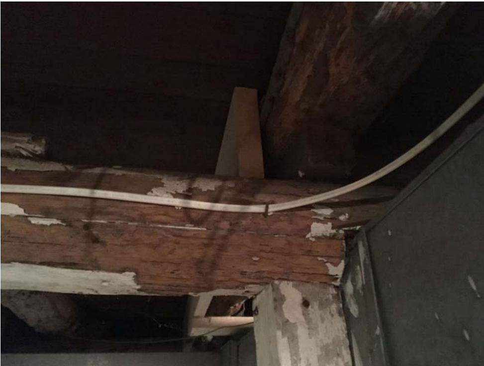
Damaged joist (main house joist)
