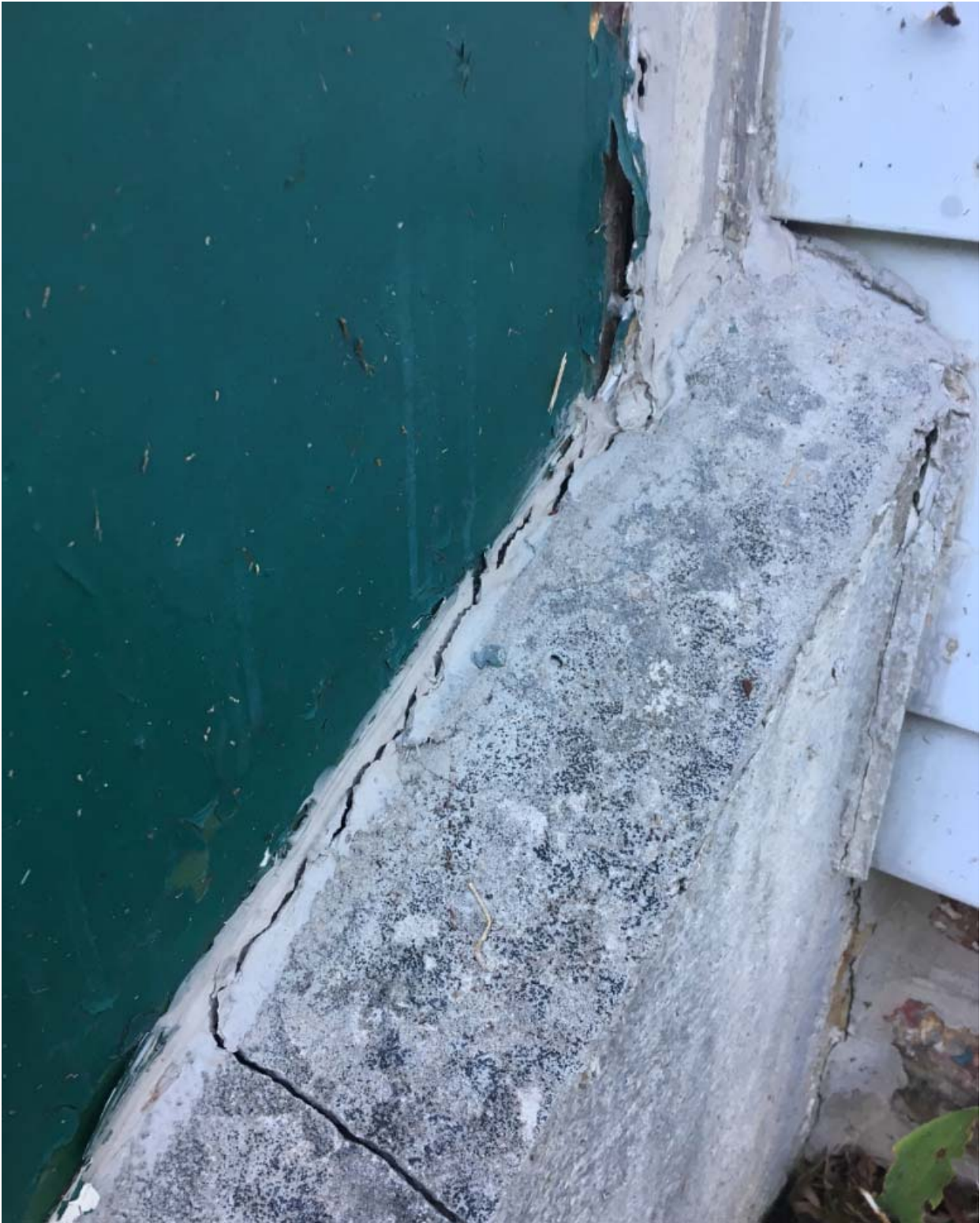
Other side of external view of cellar door. Note cracks in both caulking and mortar.
