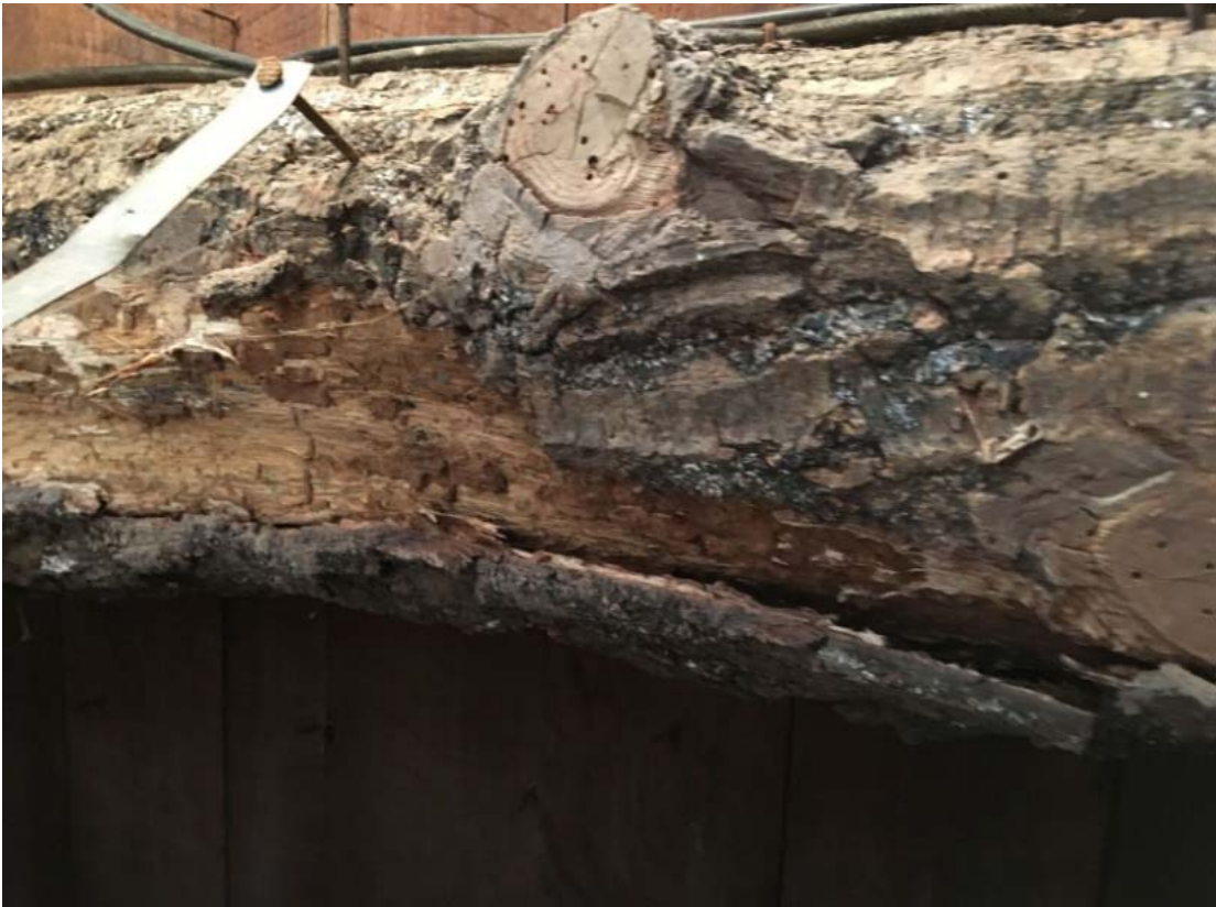
Bug damaged joist near exit
