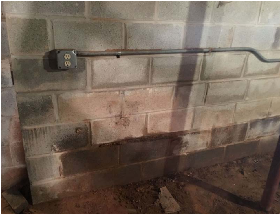
Newer wall, evidence of water
