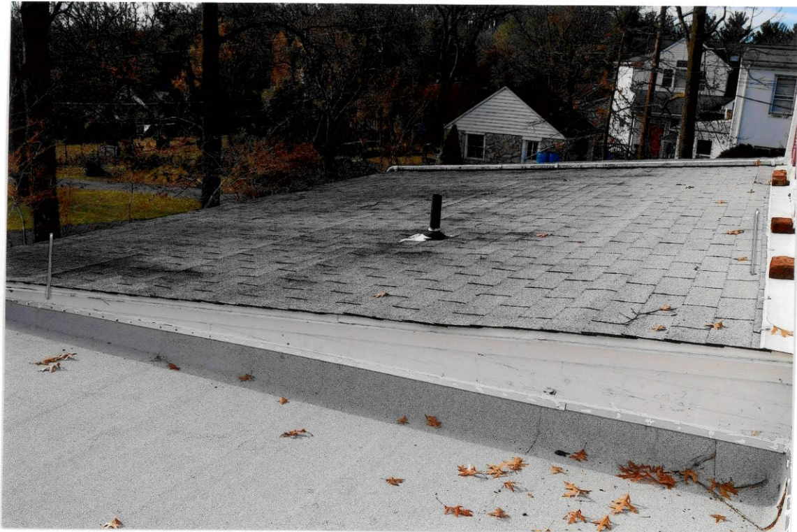
existing flat roof over kitchen has wrong type of shingles, causing leaks
