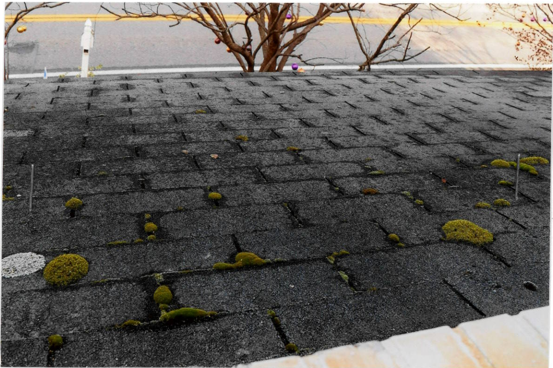
view showing poor condition of current roof
