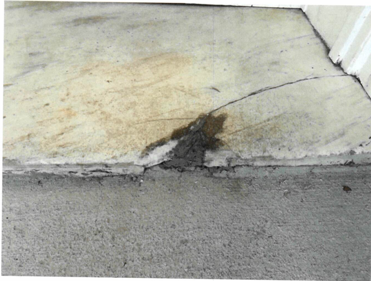
Close-up of cracked marble stoop to be repaired or replaced
