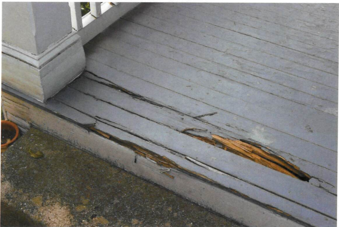
Photo 2 – Rotting floor boards
