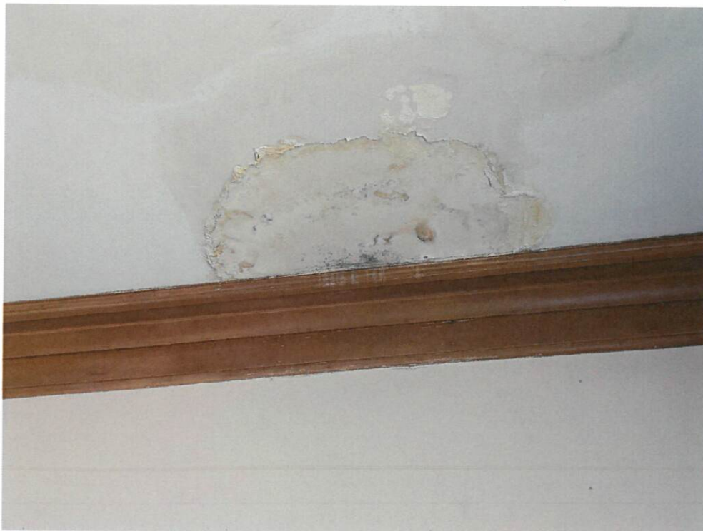
Water damage from rear porch
