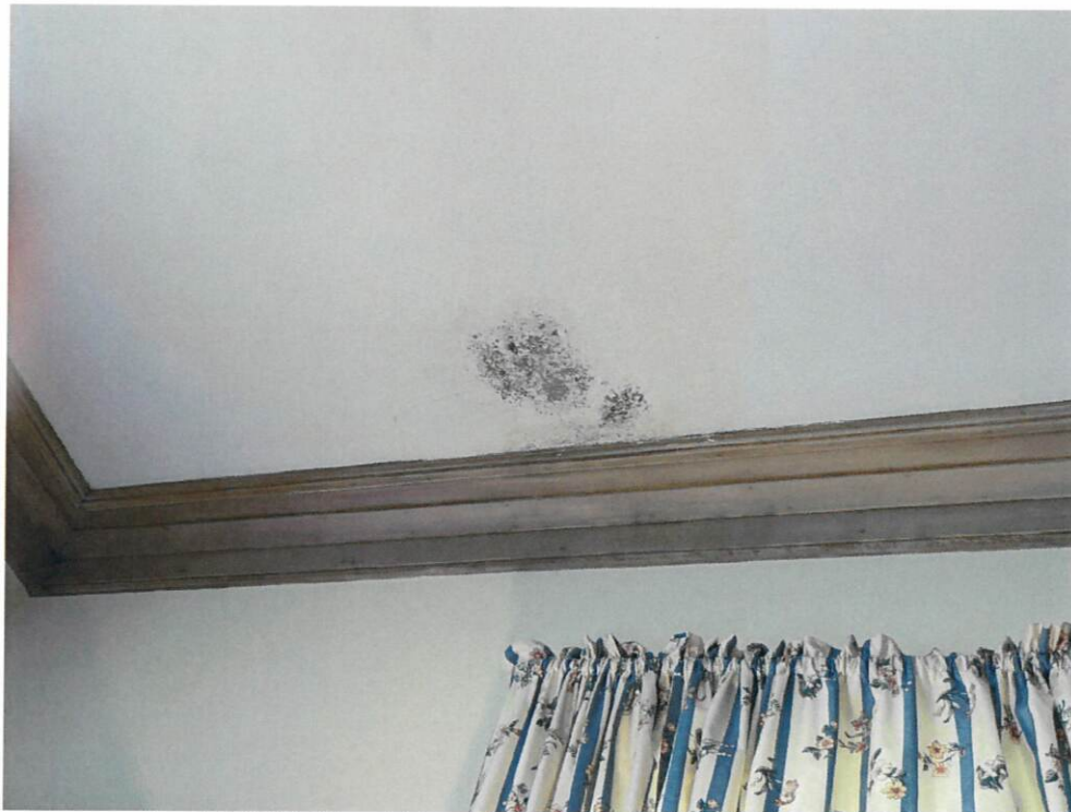
Water damage from front porch
