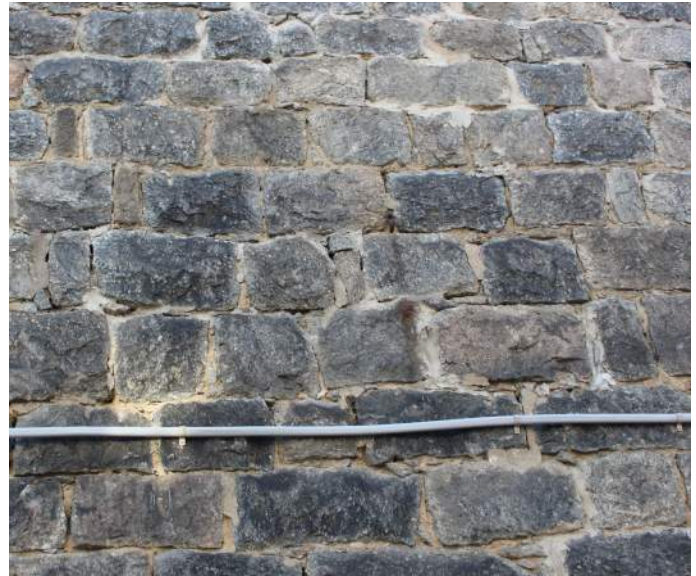
Image 5.2 - Mortar in poor condition
