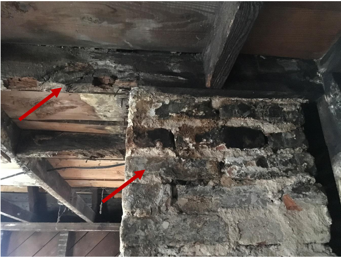
Failed joists and failing chimney
