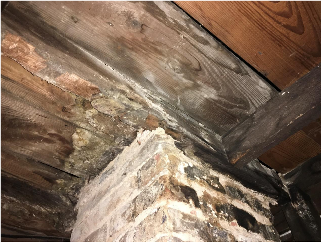
Rotten floor; Chimney in need of repair
