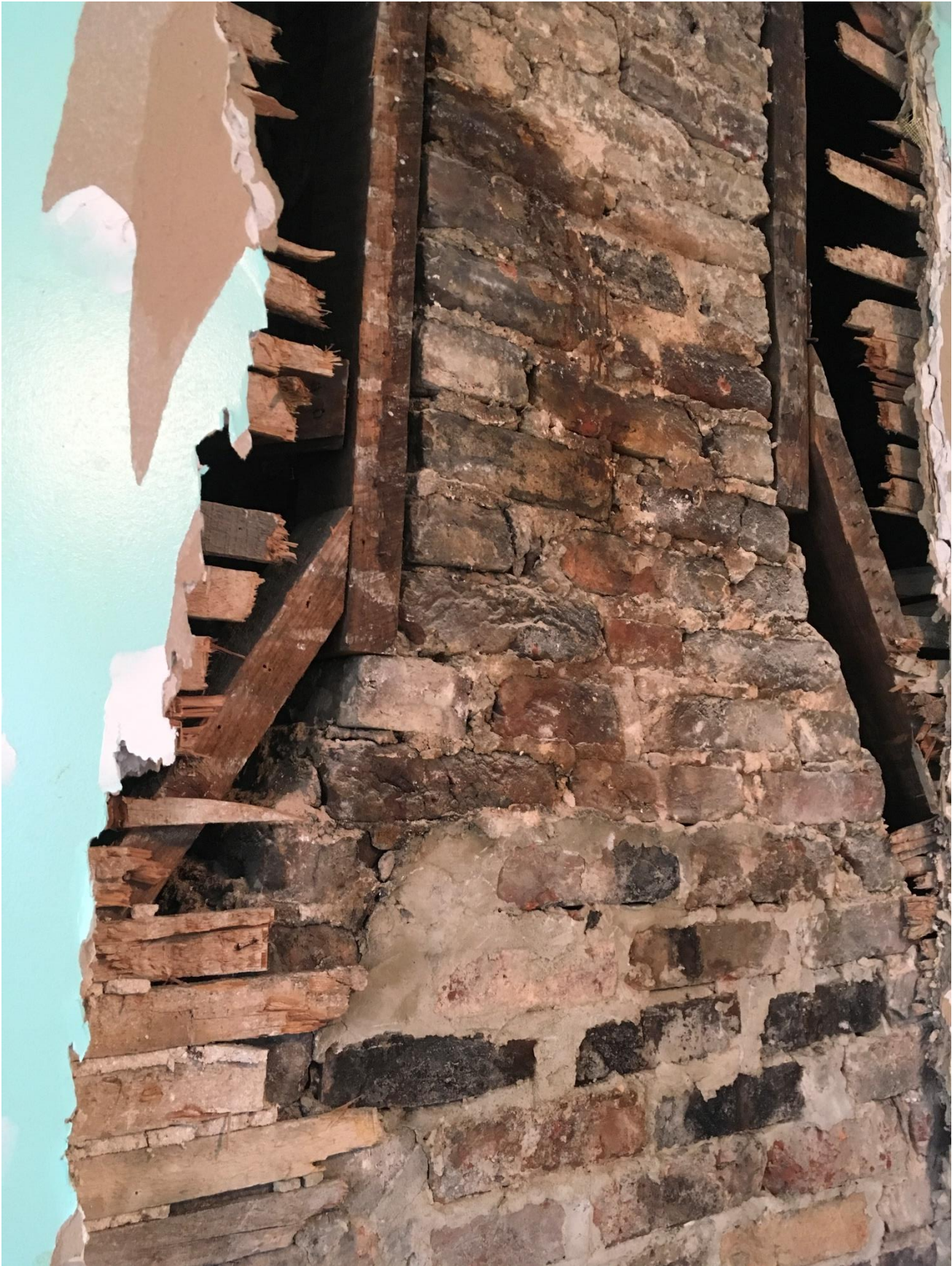
Chimney in need of repair and structural support
