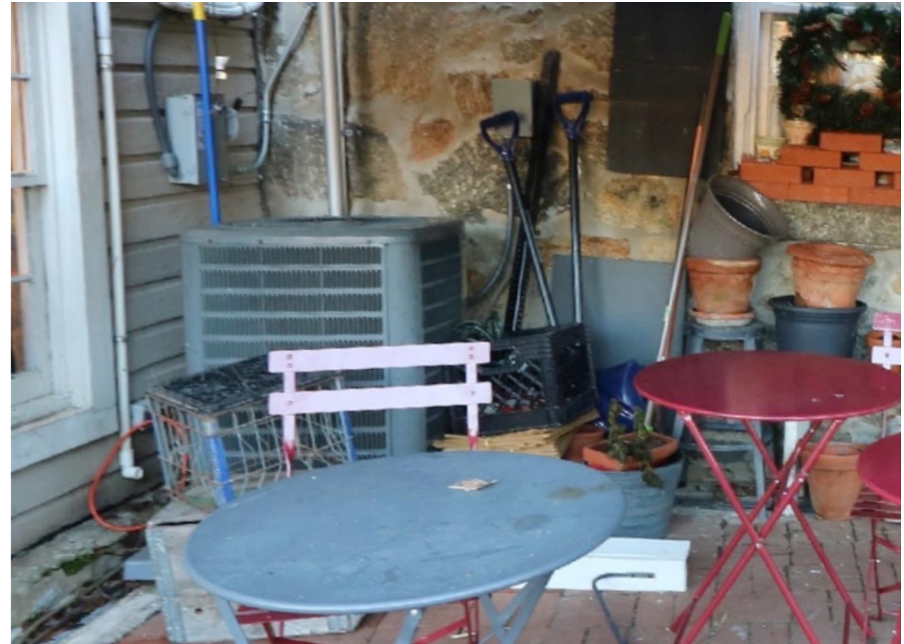
Location of AC Unit
