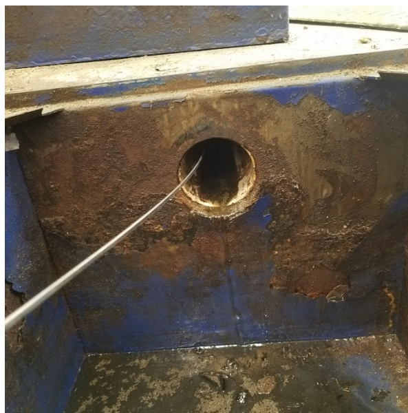
Figure 4. Inlet from floor drain.
