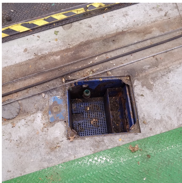
Figure 1. Oil Interceptor basin (EA3) beneath the Maintenance Shed golf cart lift.
