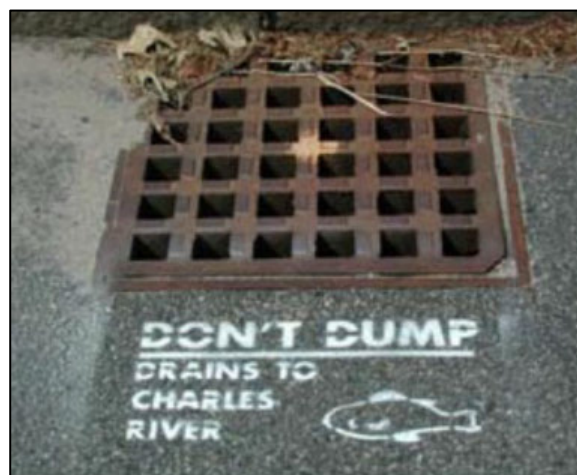
Figure 1: Storm Drain Marking
