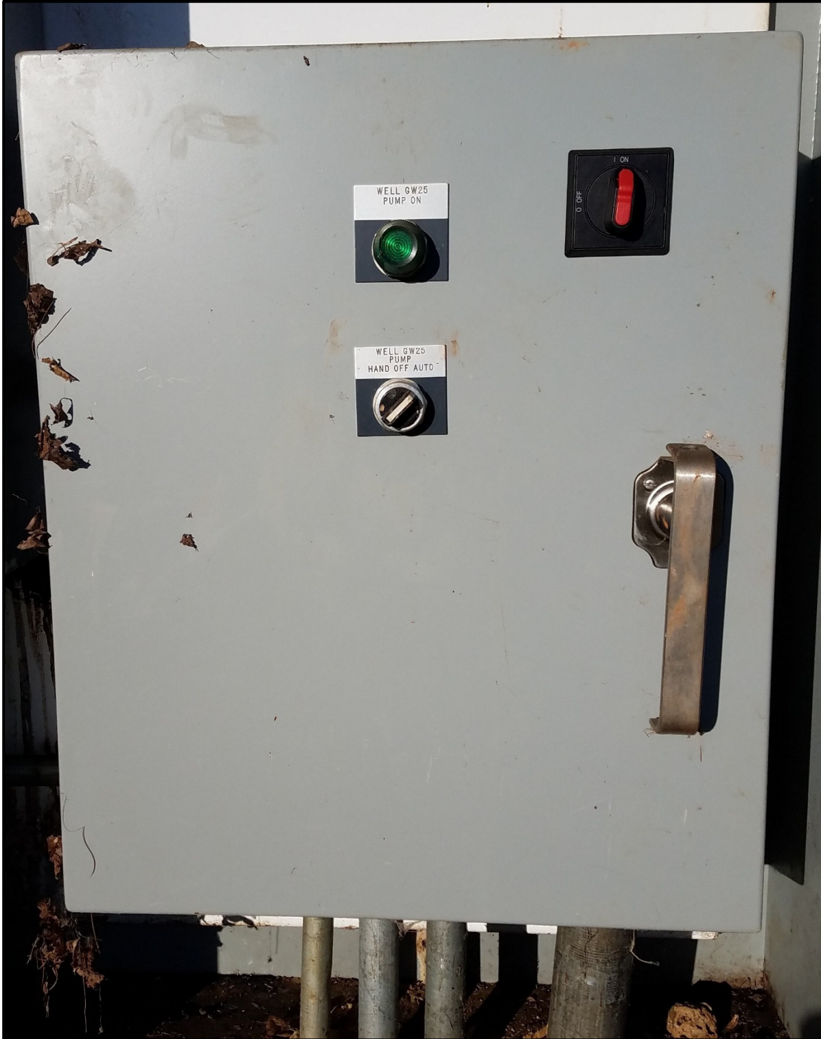
Figure 4: Alpha Ridge Landfill Well Vault Enclosure Door Outside (except wells O & P)
