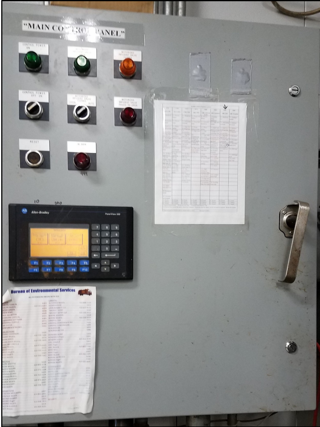
Figure 1: Alpha Ridge Landfill GWB Enclosure Door Outside
