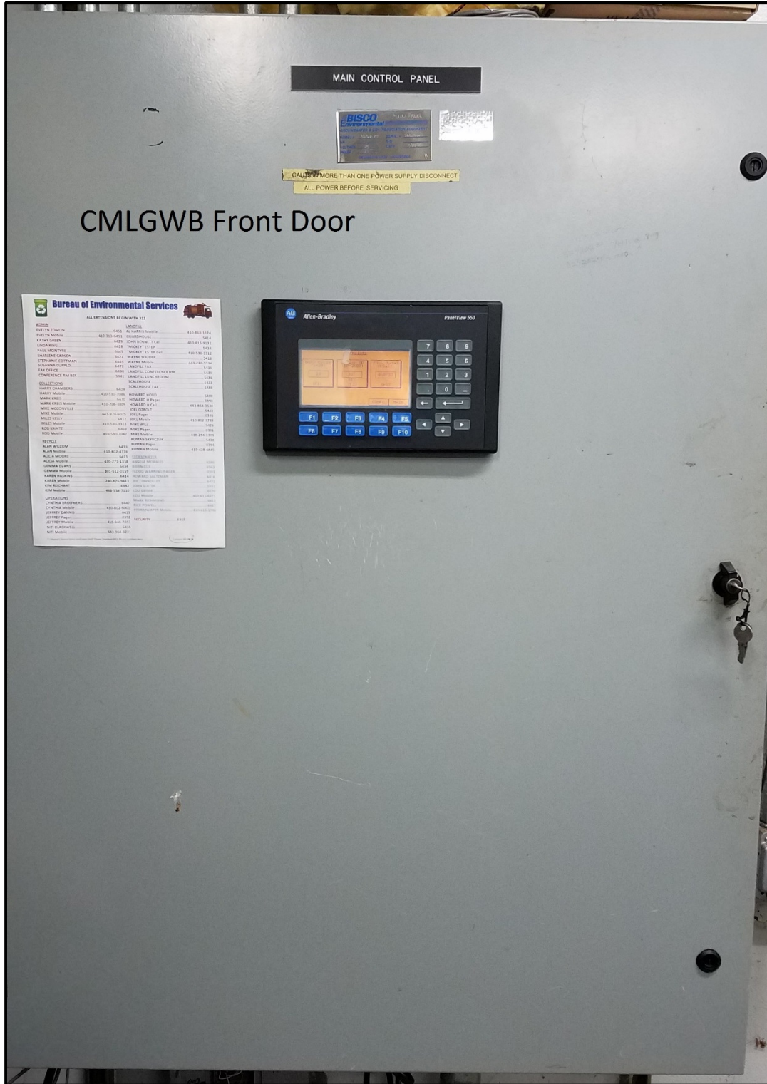
Figure 1: Carrs Mill Landfill GWB Enclosure Door Outside
