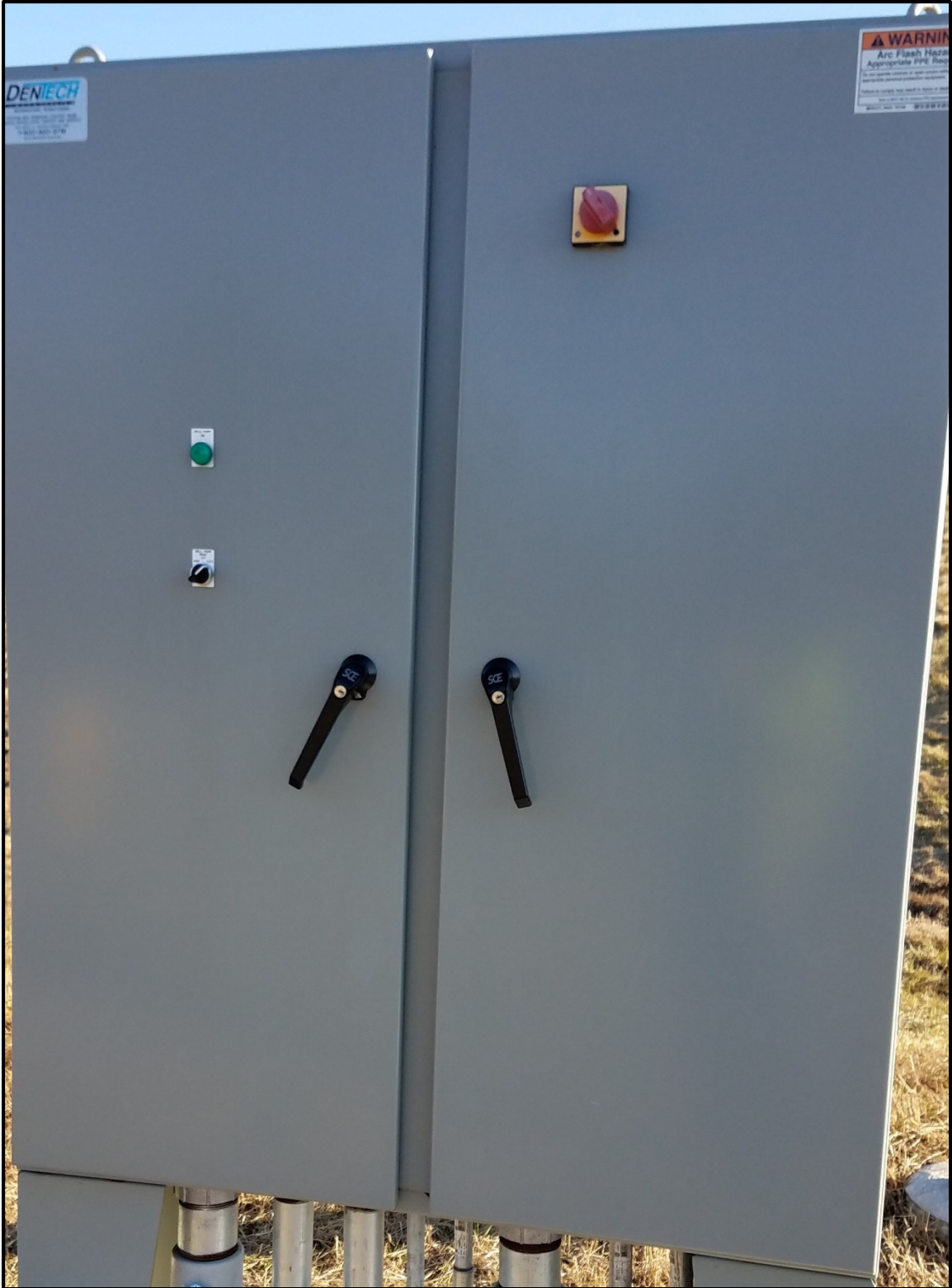
Figure 6: Alpha Ridge Landfill Well Enclosure (wells O & P)
