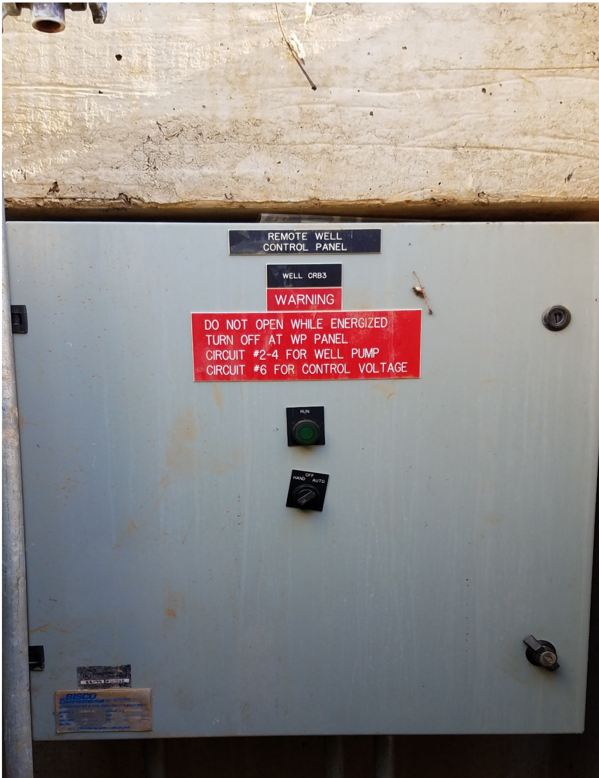
Figure 5: Carrs Mill Landfill Well Vault Enclosure Door Outside
