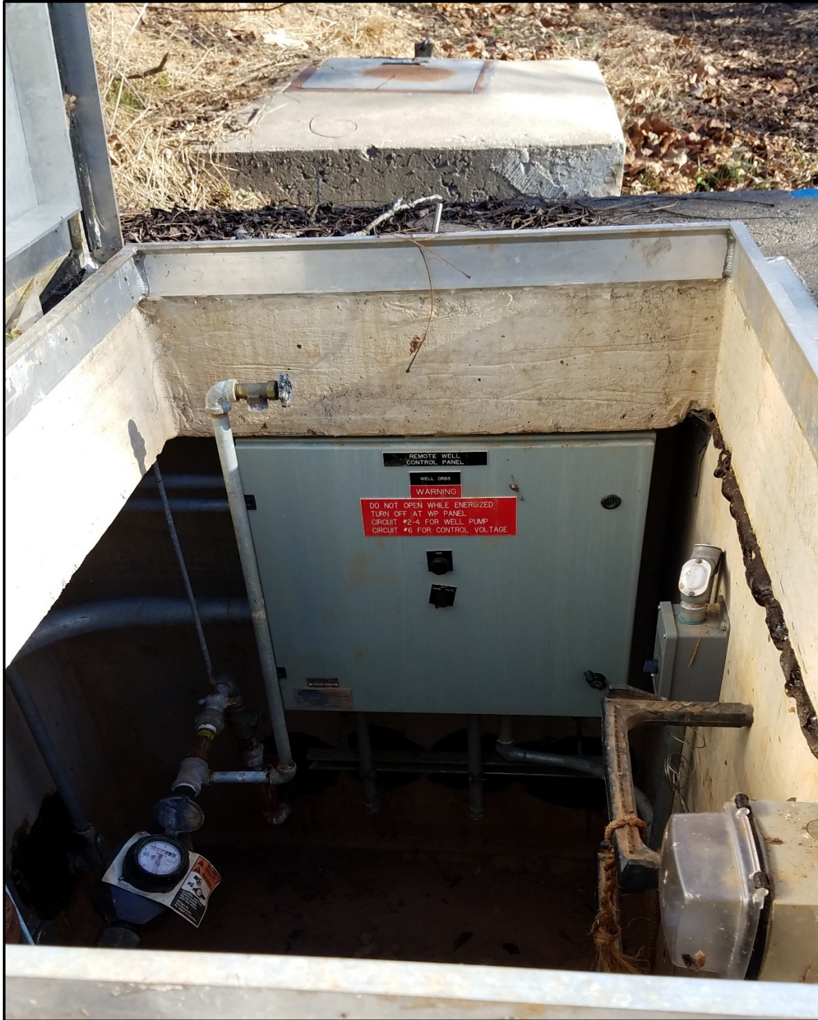
Figure 4: Carrs Mill Landfill Well Vault Panel Configuration
