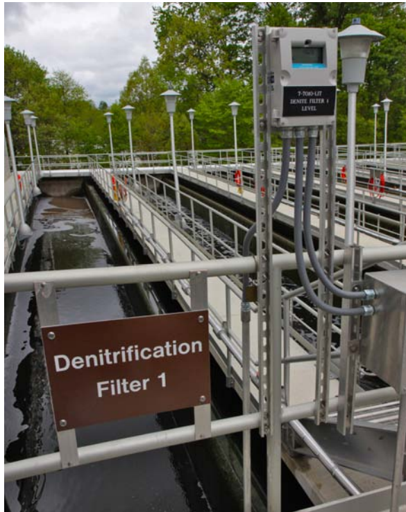
Capital investment in the County's wastewater treatment facilities is necessary for ensuring adequate capacity is available for projected population growth.
