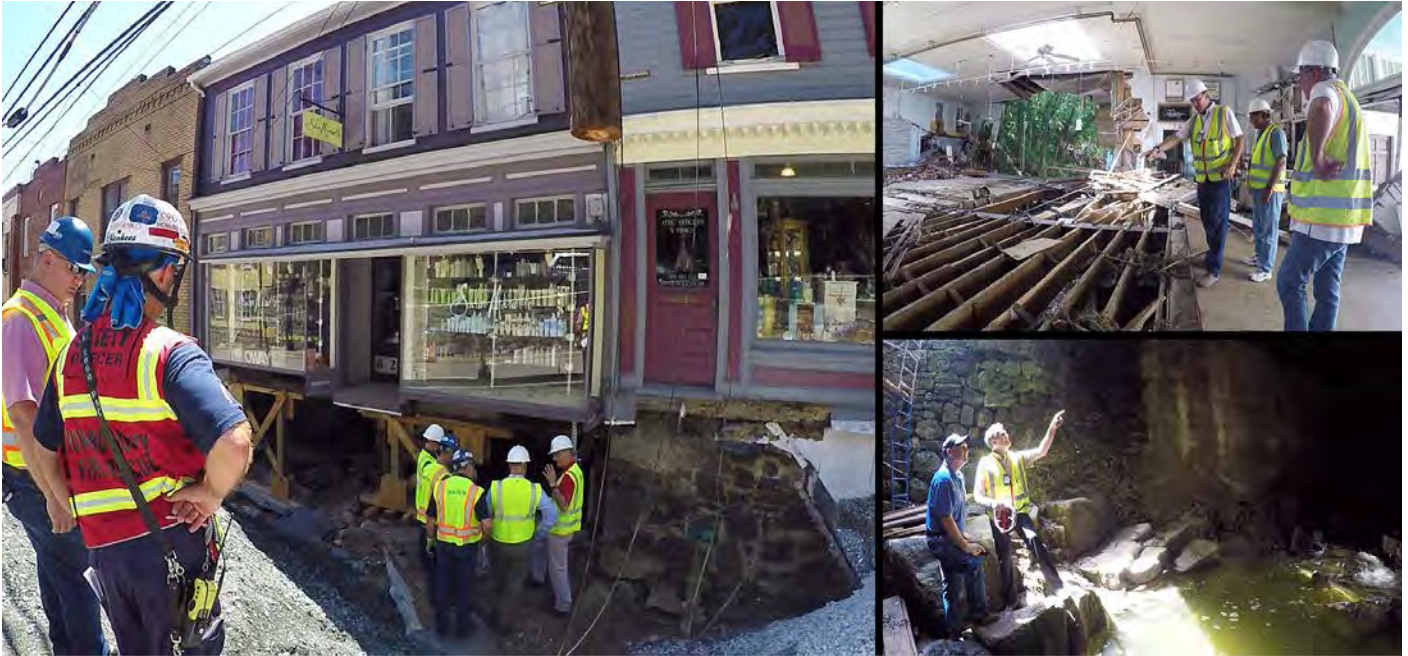
Department of Inspections, Licenses and Permits workers assess buildings damaged by the July 30th flood that devastated Historic Ellicott City.
